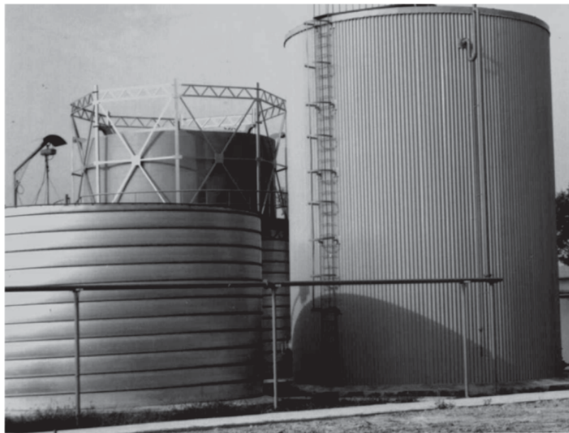
Figure 9.11 Pictorial view of anaerobic digesters.
